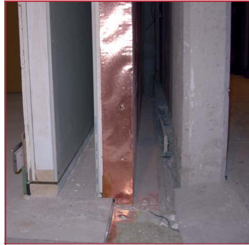
FIGURE 3. Photograph of the double casing that reduces noise transferred to the OR by the 3-T MRI machine.
